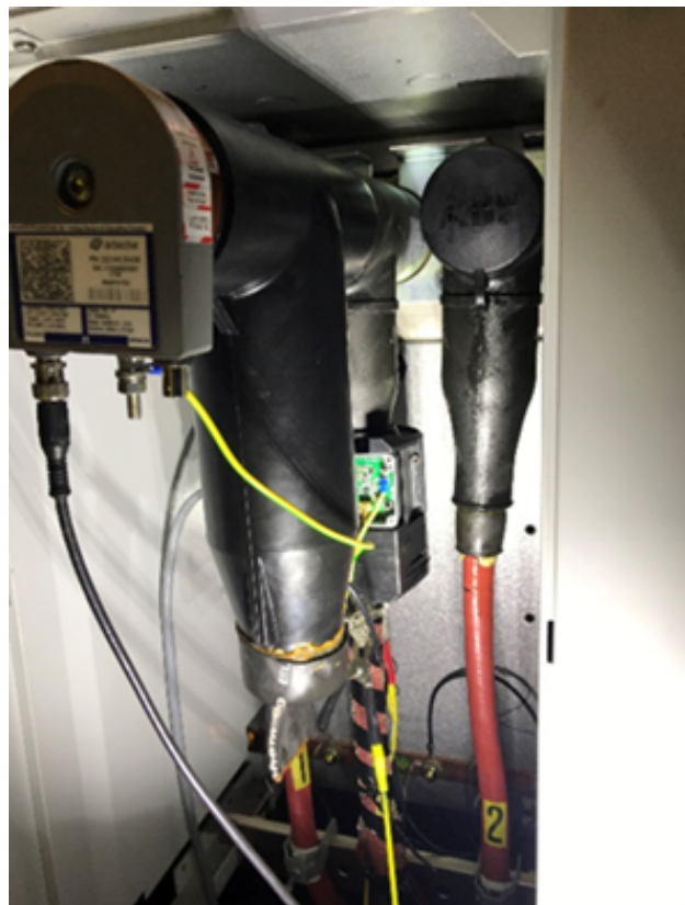
Figure 5: Sensor system installed on a single phase in the switch gear cabinet.
