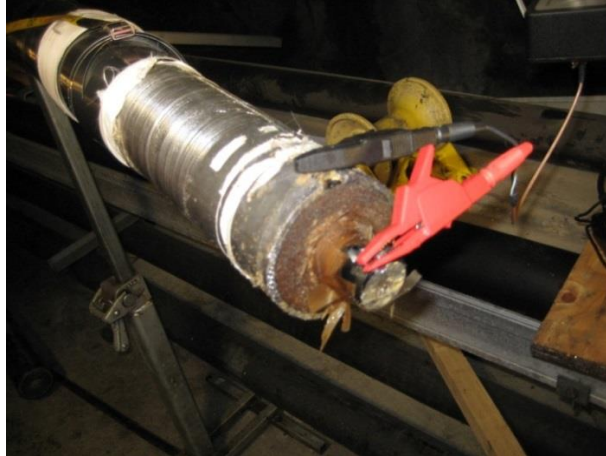
Figure 7 420 kV PILC cable with lead sheath damage
